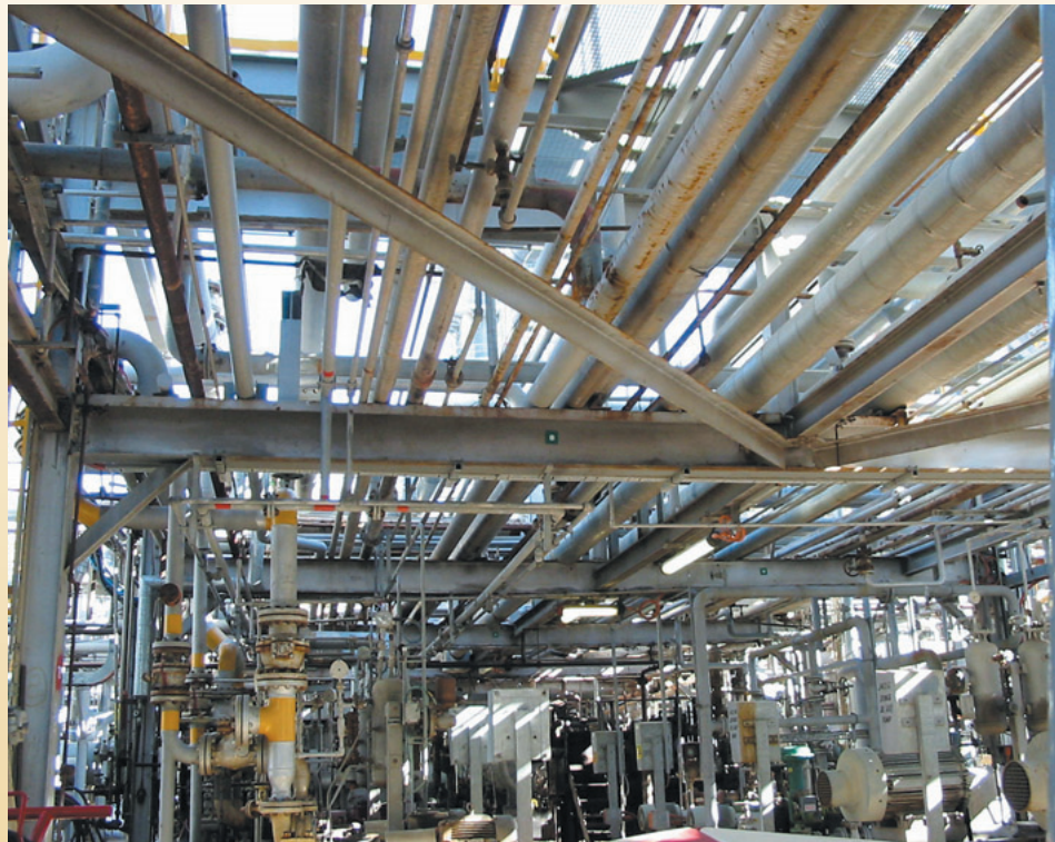
Bad as-built data can ultimately lead to longer plant shut-downs.
